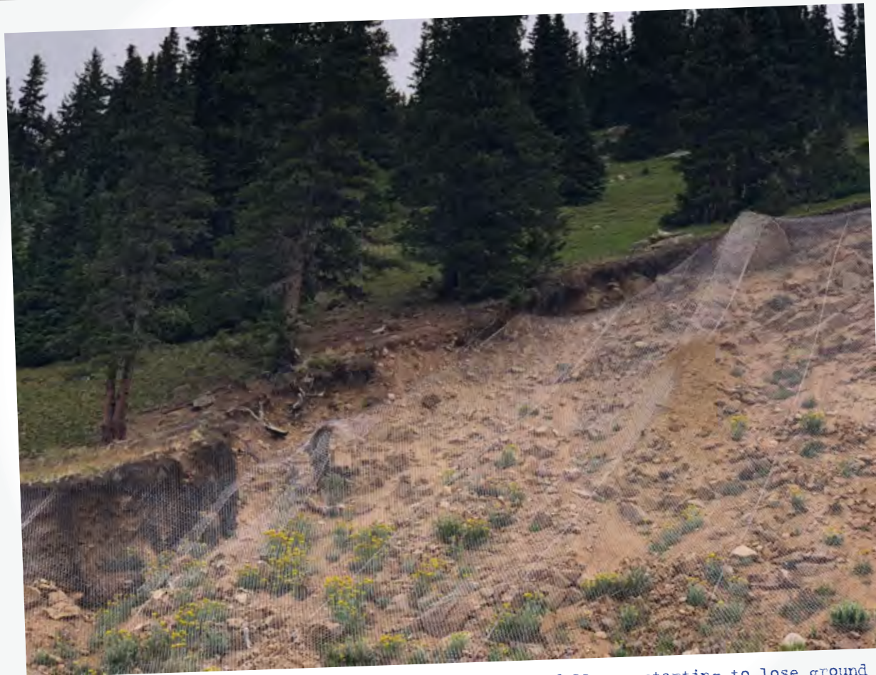
Metal nets installed in the mid-2000s to retard rockfall are starting to lose ground
